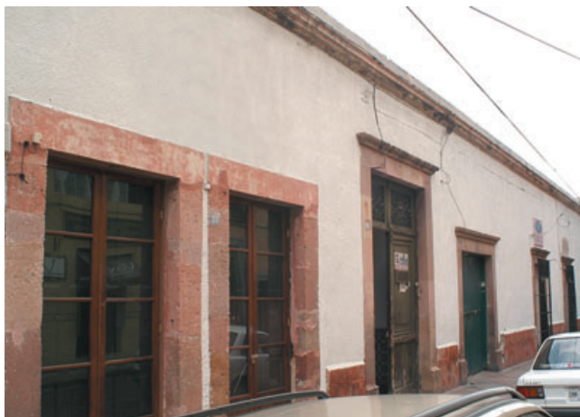
Figure 3 Photograph of the frontage of El Museo del Calendario, showing the conservation state before the restoration process.
